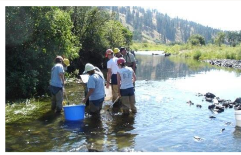
Crews catch and relocate fish to prevent them from being impacted by construction of a restoration project. 9
